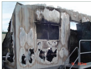
Fire damage in Illinois
