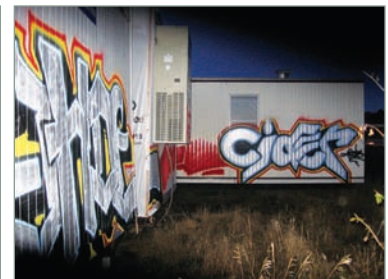
Graffiti damage in Minnesota
