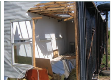
Hurricane Ike damage in Texas
