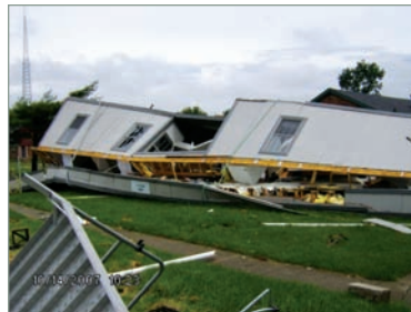
Tornado damage in Indiana
