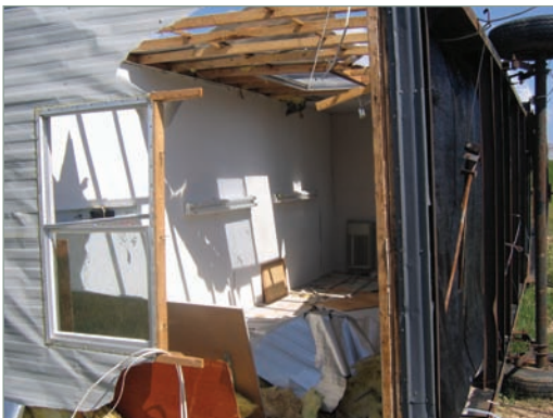
Hurricane Ike damage in Texas
